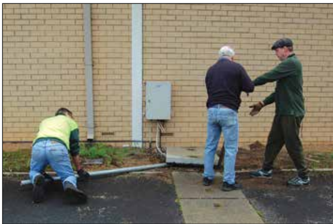
Nick Daniele and Ron Fabry levering the concrete slab back into place at the main building end of the trench as Chad Raven steps in to save Ron's back.
